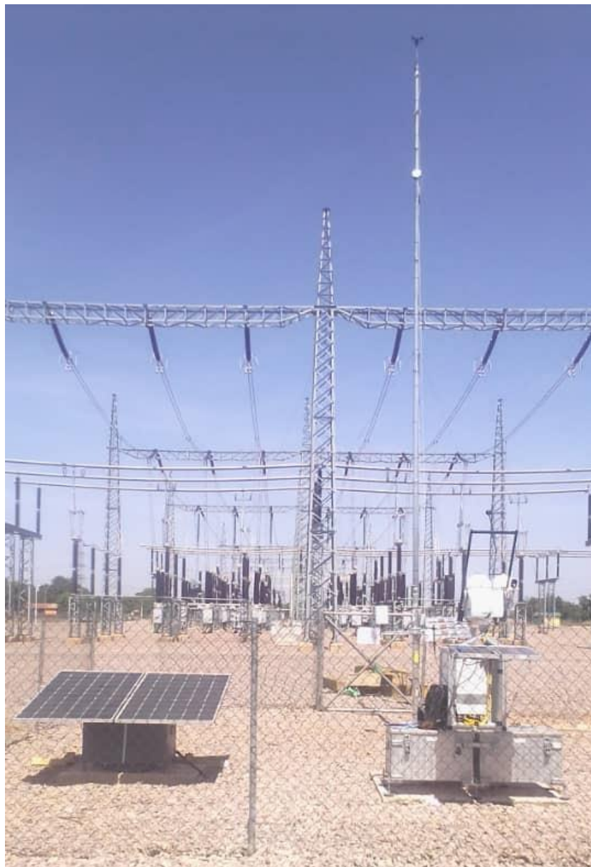
Figure 41 : Installation finale de la station vue du sud / Final station installation as seen from south.
