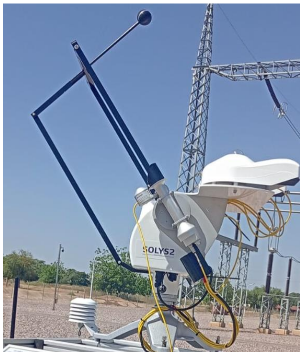
Figure 22 : Tracker installé / Installed tracker
