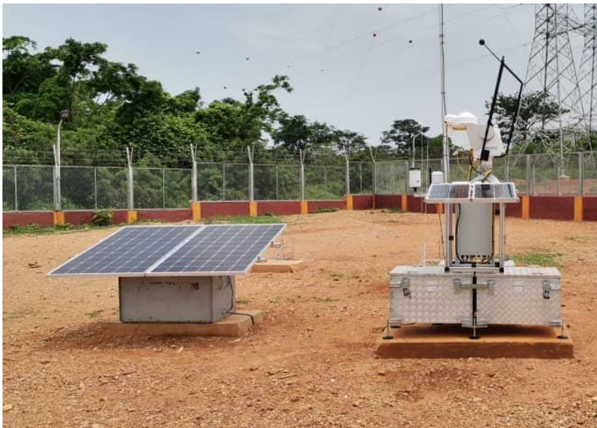
Figure 41 : Installation finale de la station vue du sud / Final station installation as seen from south
