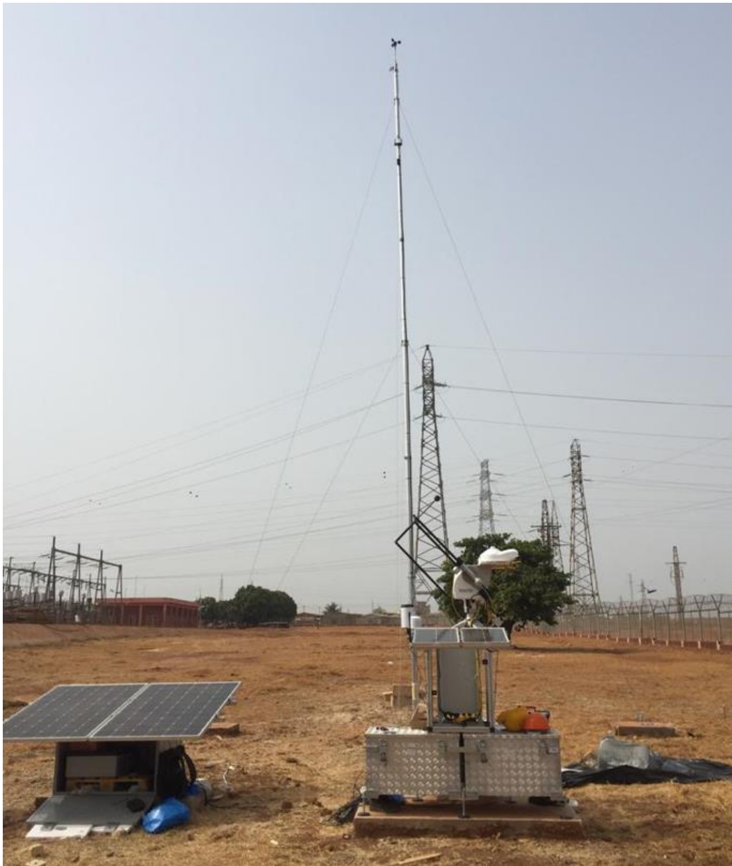
Figure 76 : Installation de la station vue du sud / Station installation as seen from south.
