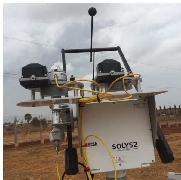
Figure 57 : Tracker installé / Installed tracker.
