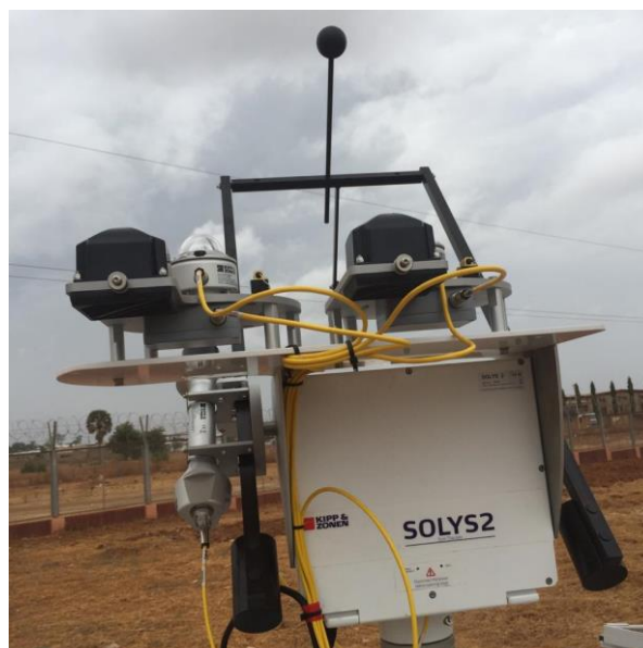
Figure 22 : Tracker installé / Installed tracker
