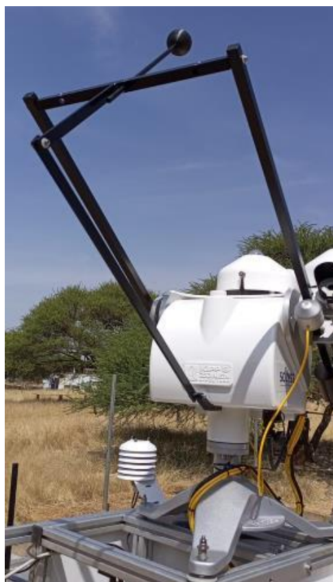
Figure 57: Tracker installé / Installed tracker.
