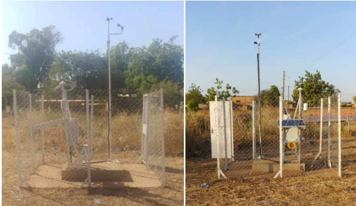
Figure 9: Station Tier2 comme installée à Kaya, Burkina Faso / Tier2 station as installed in Kaya, Burkina Faso.
