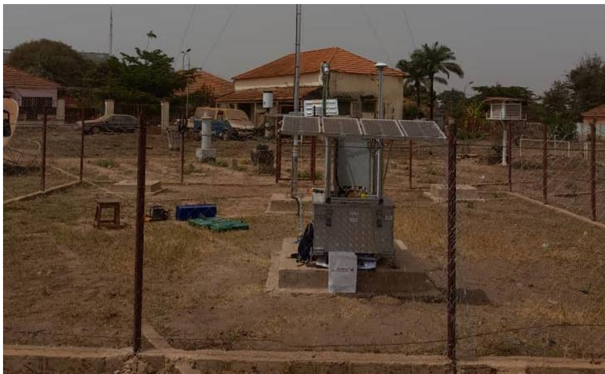
Figure 37 : Installation finale de la station depuis le sud / Final station installation from south
