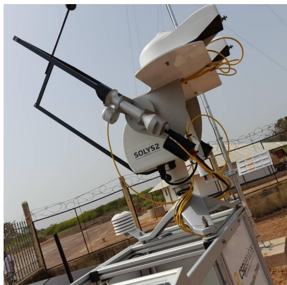
Figure 57: Tracker installé / Installed tracker.
