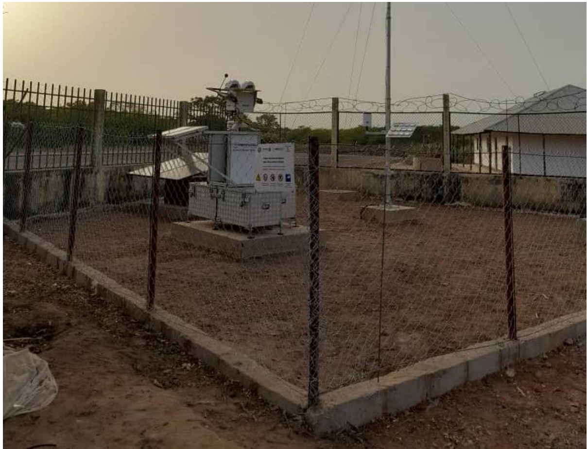
Figure 75 : Installation finale de la station vue du sud-est / Final station installation as seen from south-east.
