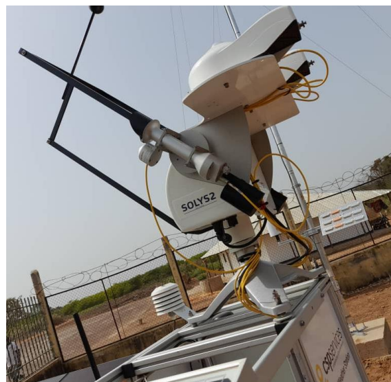
Figure 22 : Tracker installé / Installed tracker
