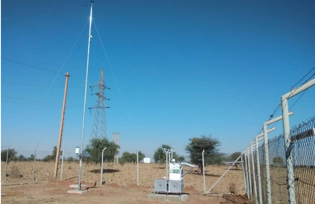
Figure 36 : Installation finale de la station depuis le sud-ouest / Final station installation from southwest
