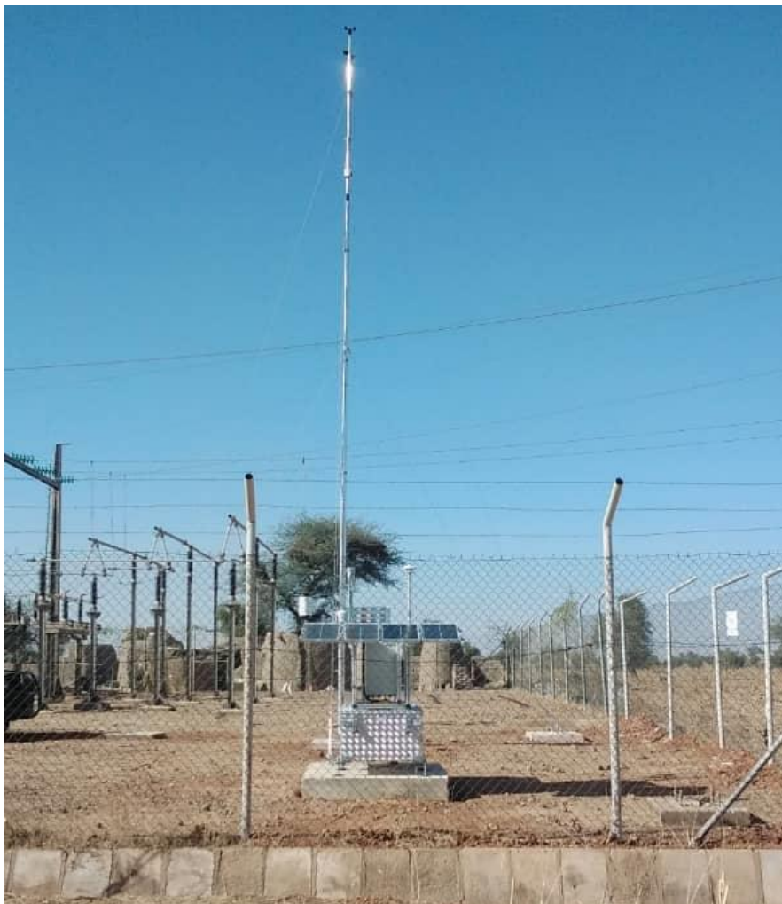
Figure 37 : Installation finale de la station depuis le sud / Final station installation from south
