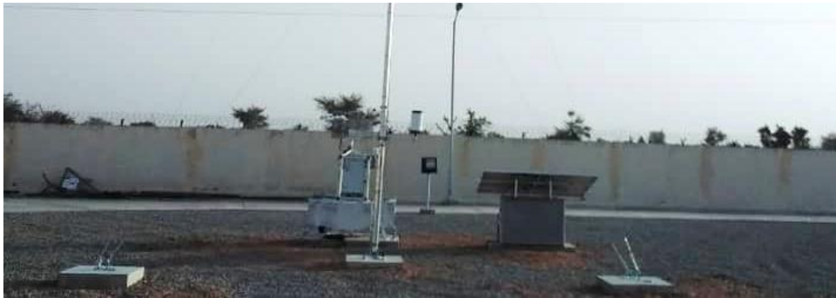
Figure 40 : Installation finale de la station vue du nord/ Final station installation as seen from north
