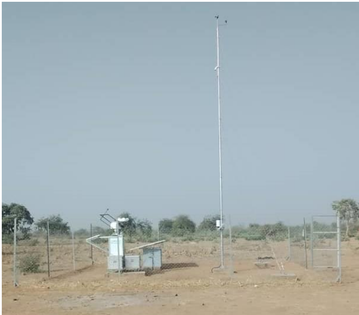
Figure 41 : Installation finale de la station vue d'est / Final station installation as seen from east
