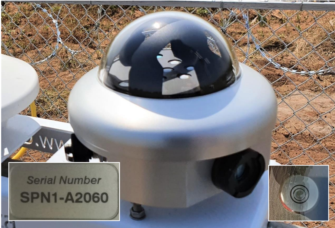
Figure 9: DHI Pyranometer Installation
