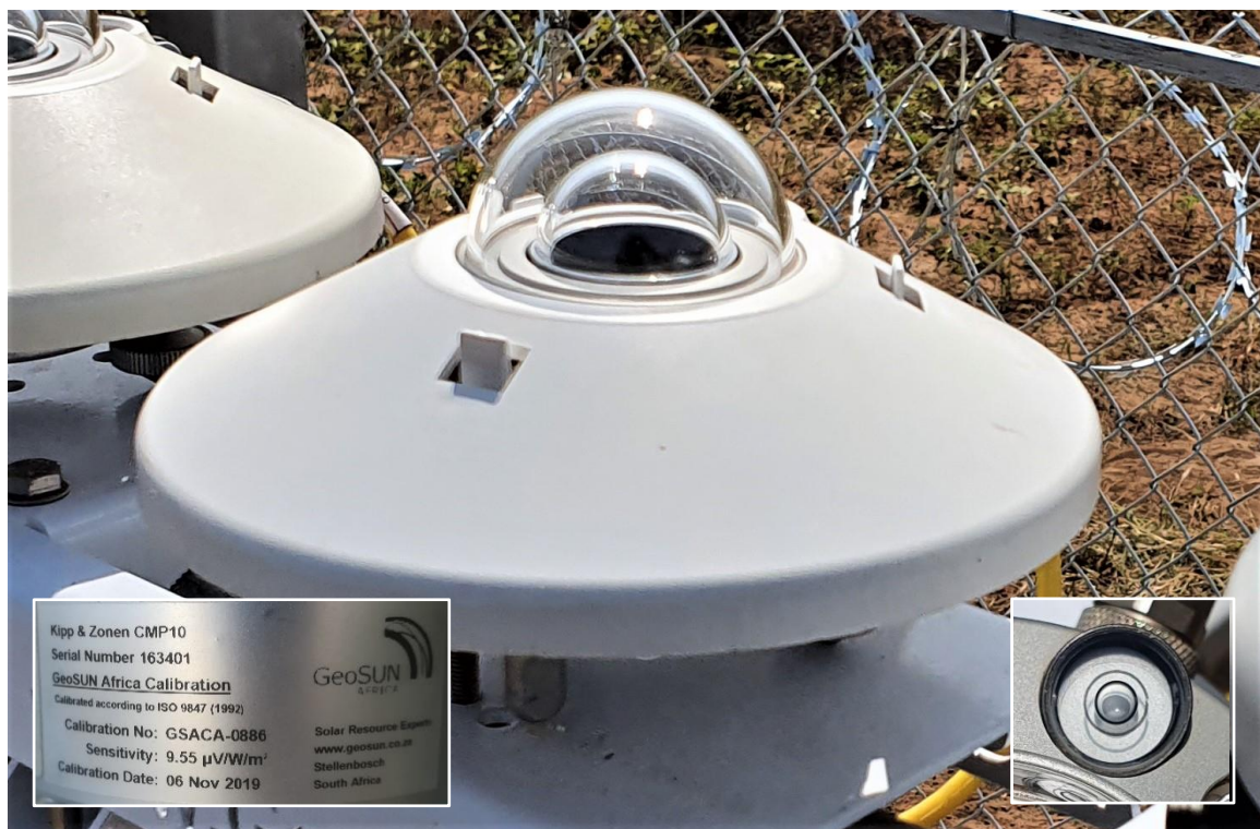
Figure 8: GHI (2) Pyranometer Installation
