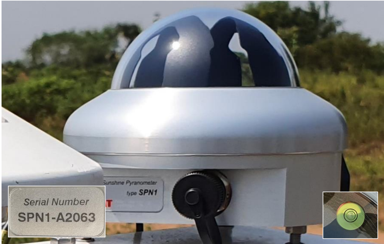
Figure 9: DHI Pyranometer Installation
