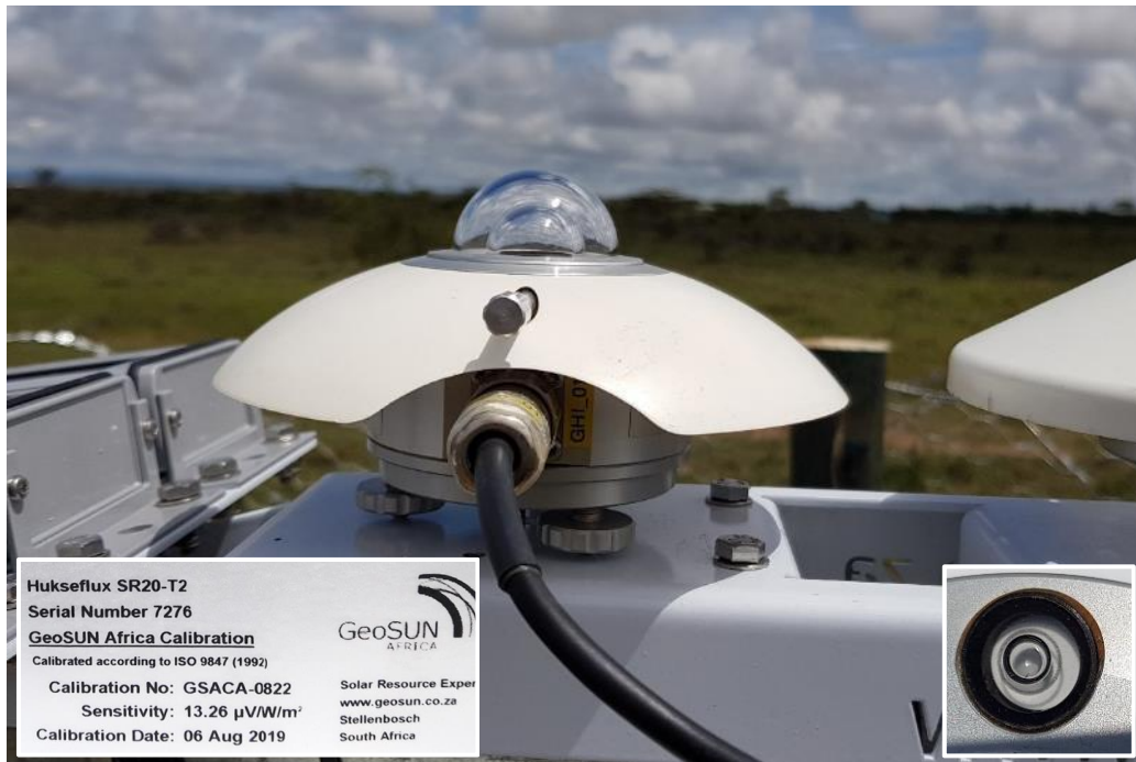
Figure 7: GHI (1) Pyranometer Installation
