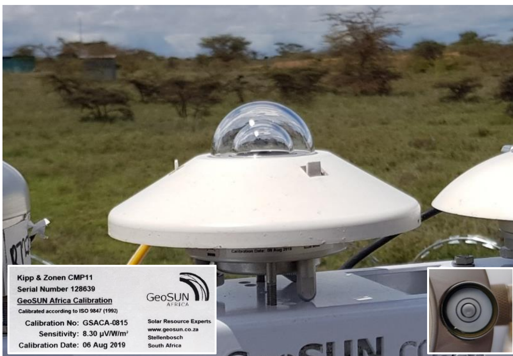
Figure 8: GHI (2) Pyranometer Installation
