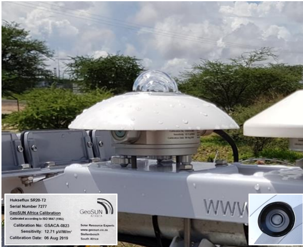
Figure 7: GHI (1) Pyranometer Installation
