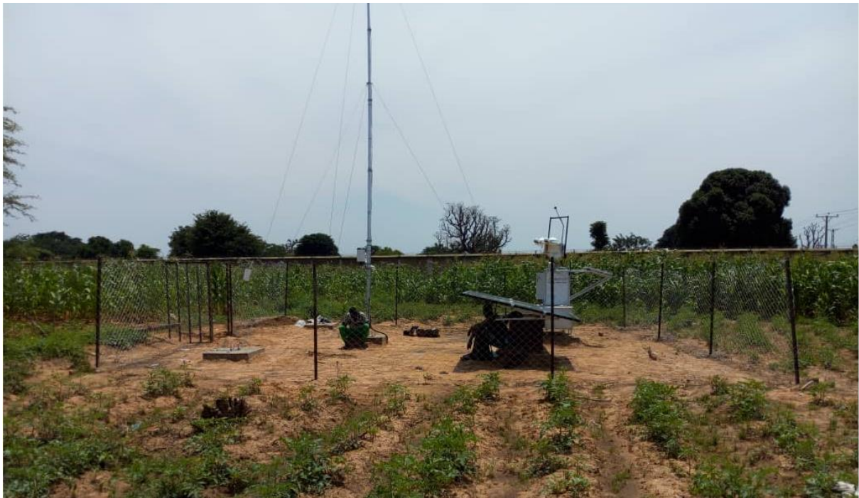
Figure 39 : Installation finale de la station vue de l'ouest / Final station installation as seen from west
