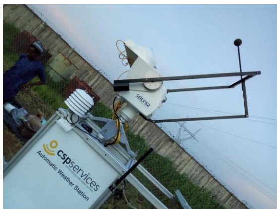
Figure 57 : Tracker installé / Installed tracker.
