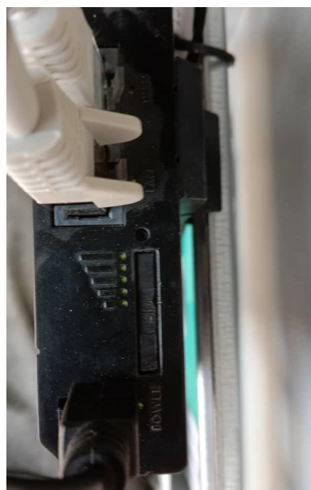
Figure 100: Vérification de la communication du modem / Modem communication check.
