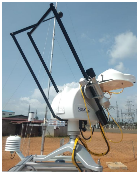
Figure 22 : Tracker installé / Installed tracker
