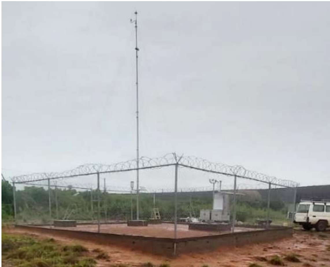
Figure 42 - Site with completed station installation as seen from south-west. Picture taken from 6.49767°N, -10.65176°E
