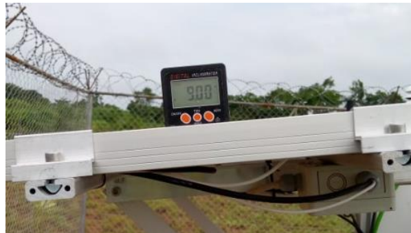
Figure 34 - PV-S support structure with 9° tilt angle towards South
