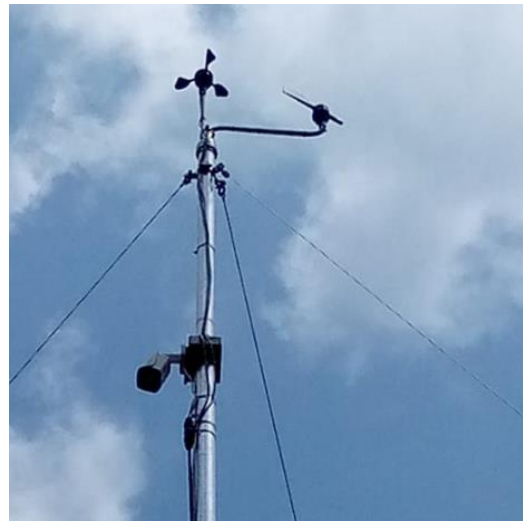
Figure 16 - Wind sensors installed on wind mast
