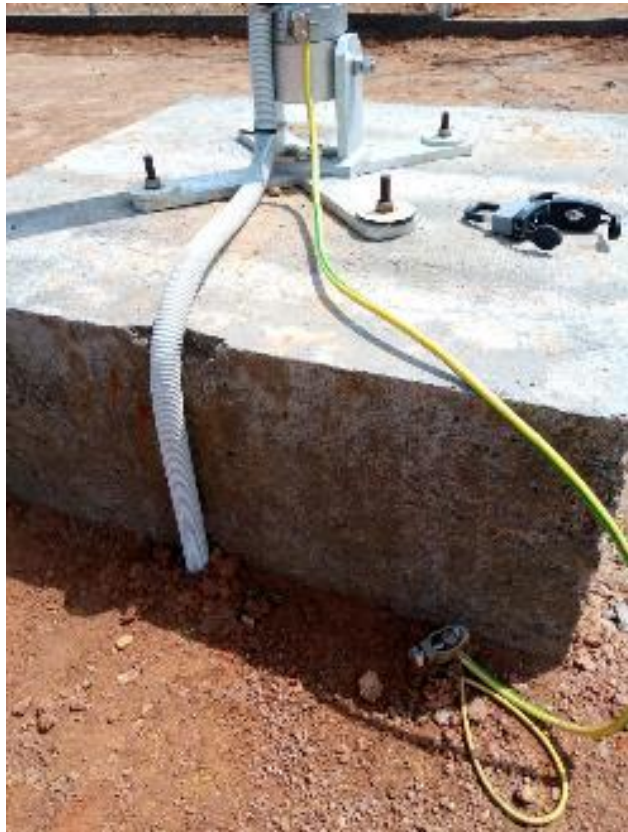
Figure 12 - Wind mast foundations, ground cable fixed to ground bolt, protective tube for wind mast cables.
