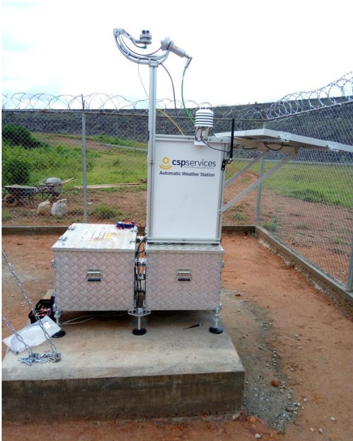
Figure 40 - Main mounting structure with solar sensors, T/RH sensor and PV panels for soiling measurement and power supply.
