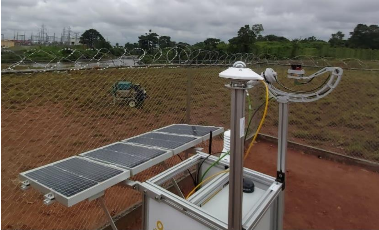
Figure 41 - Solar sensors and PV panels on mounting structure
