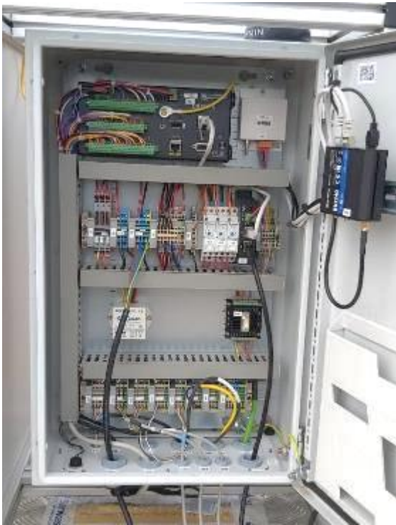
Figure 31 - Control box interior; top: datalogger; bottom: fuses and 12V circuit distribution, relays, RSI motor controller
