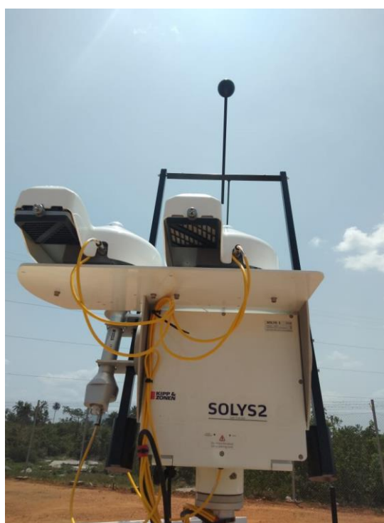
Figure 57 : Tracker installé / Installed tracker.
