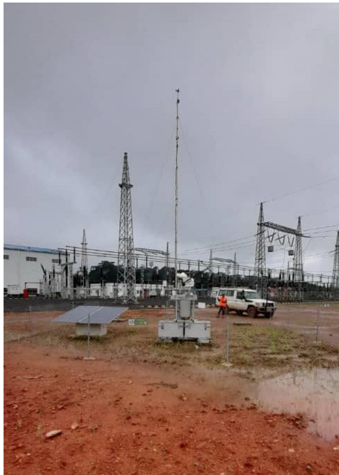
Figure 91 : Vue générale de la station / General view of the station.
