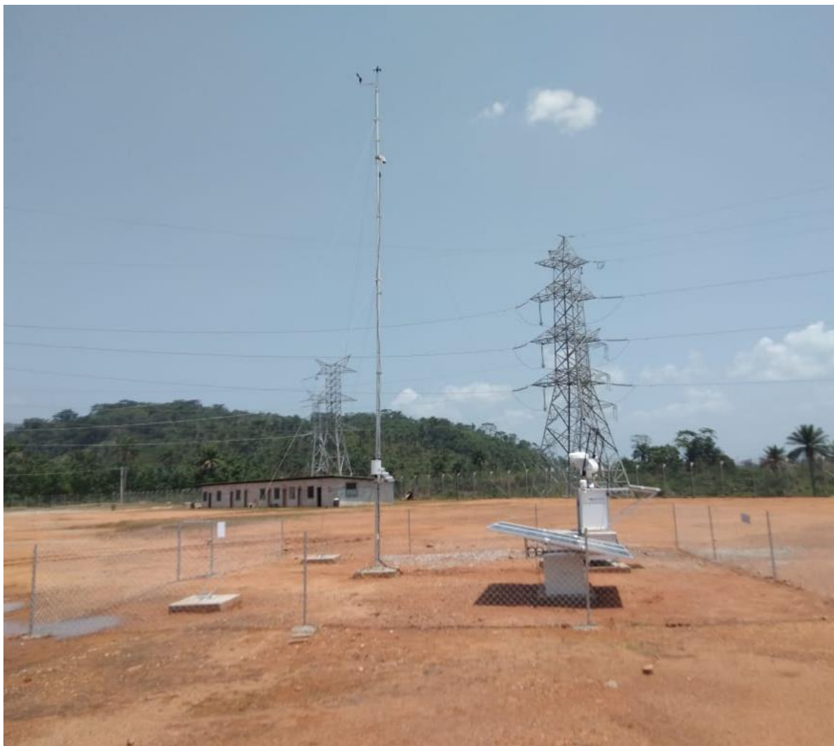
Figure 76 : Installation finale de la station vue d'ouest / Final station installation as seen from west.
