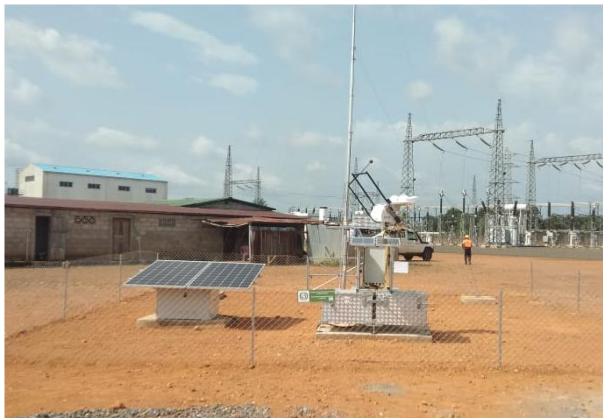
Figure 76 : Installation finale de la station vue du sud / Final station installation as seen from south.
