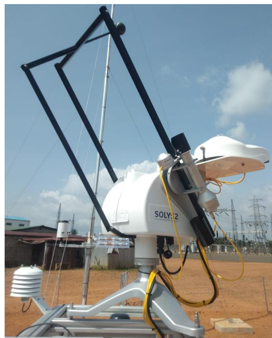
Figure 57 : Tracker installé / Installed tracker.
