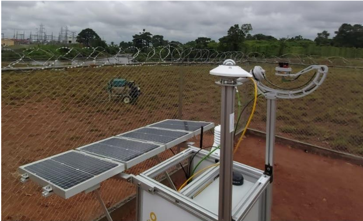
Figure 73 - Solar sensors and PV panels on mounting structure
