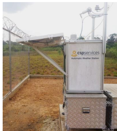
Figure 89: Station structure with PV modules
