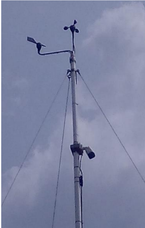
Figure 76: Wind mast top section with sensors and camera
