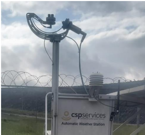
Figure 107: T/RH sensor and modem antenna on the station mounting structure
