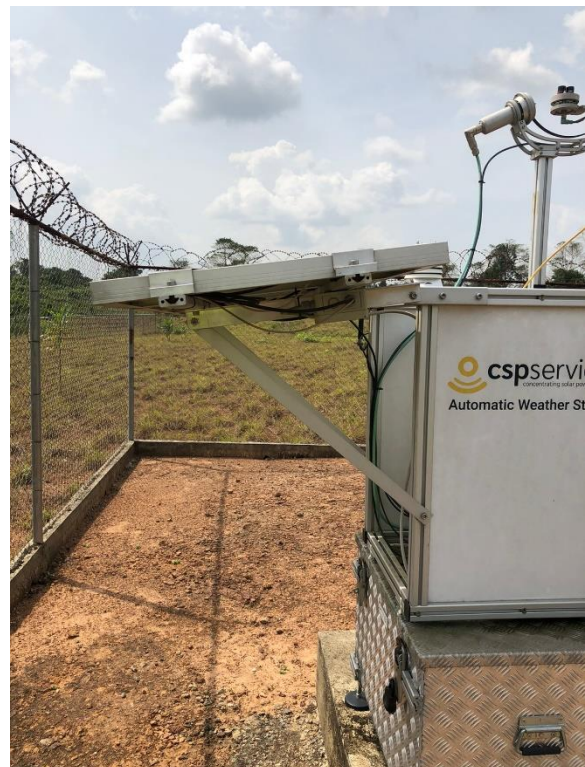
Figure 130: Station structure with PV modules
