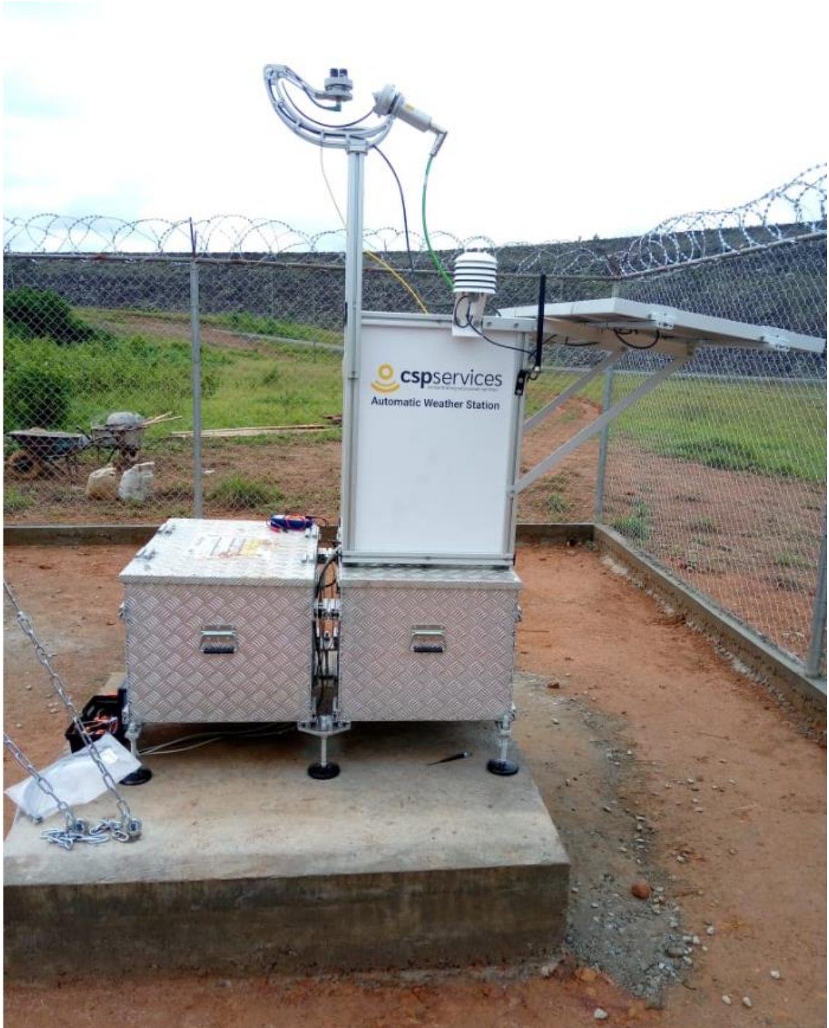
Figure 72 - Main mounting structure with solar sensors, T/RH sensor and PV panels for soiling measurement and power supply.
