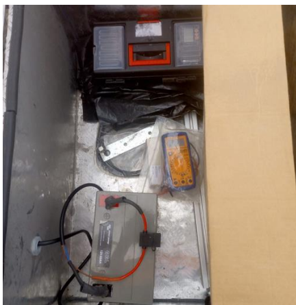
Figure 88: Battery box interior
