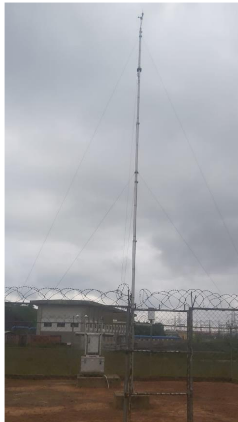
Figure 98: Wind mast with foundations and guying ropes
