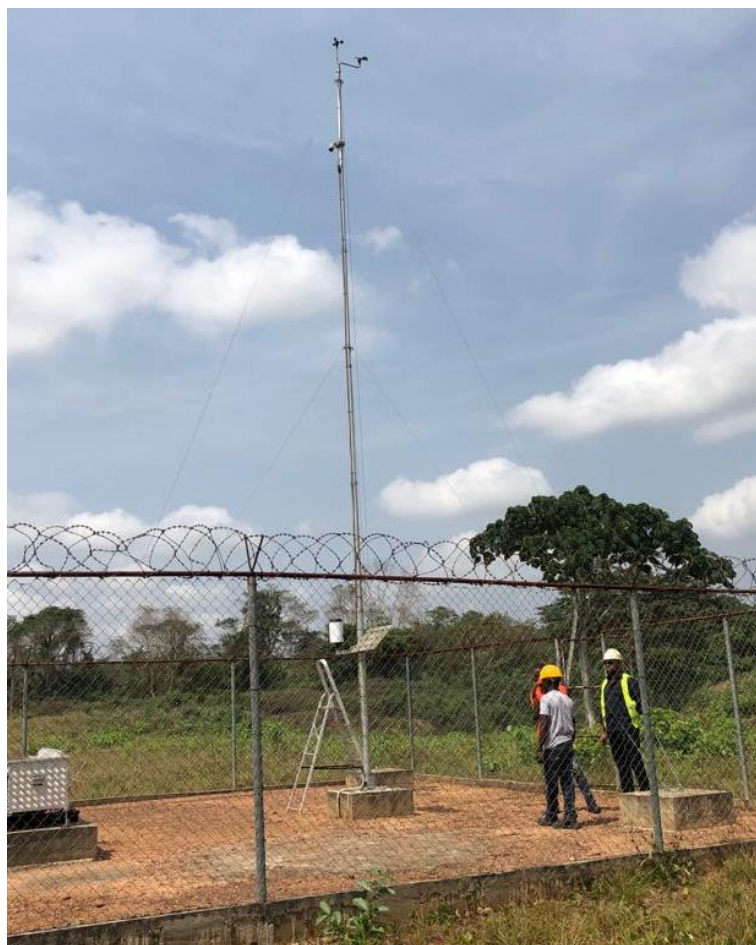
Figure 118: Wind mast with foundations and guying ropes
