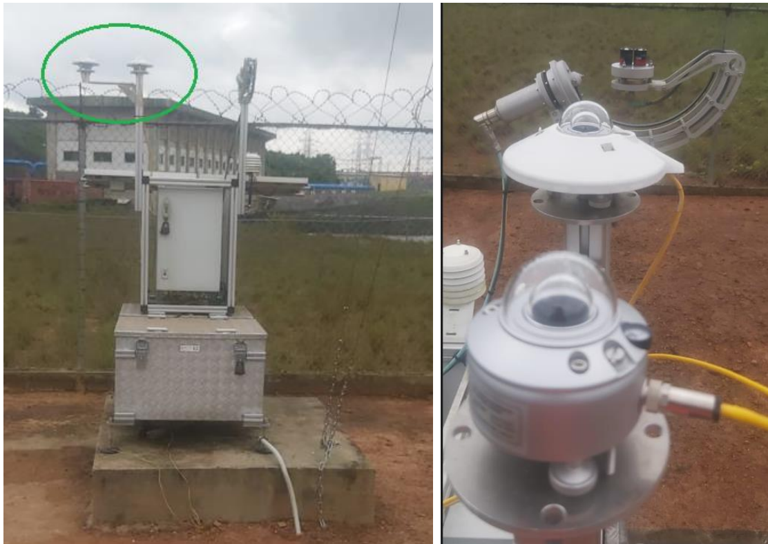
Figure 139: Reference pyranometer installation
