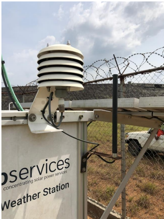
Figure 127: T/RH sensor and modem antenna on the station mounting structure
