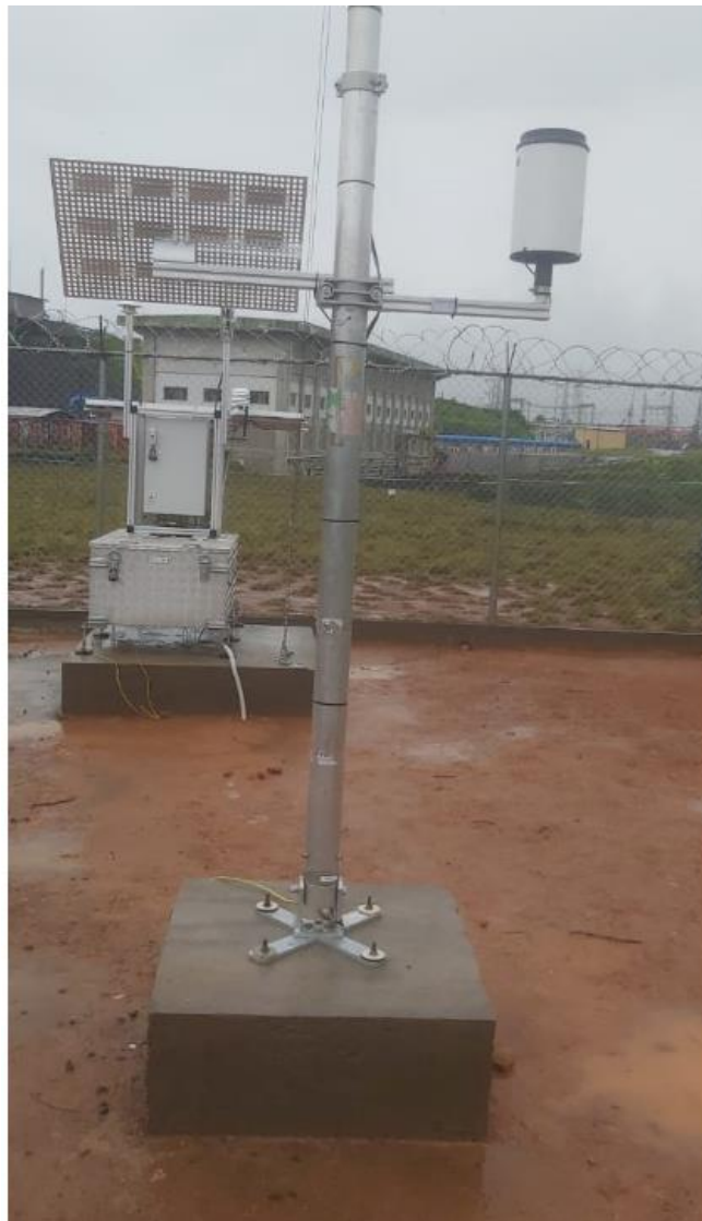
Figure 71 - Wind mast with rain sensor and corrosion sampler
