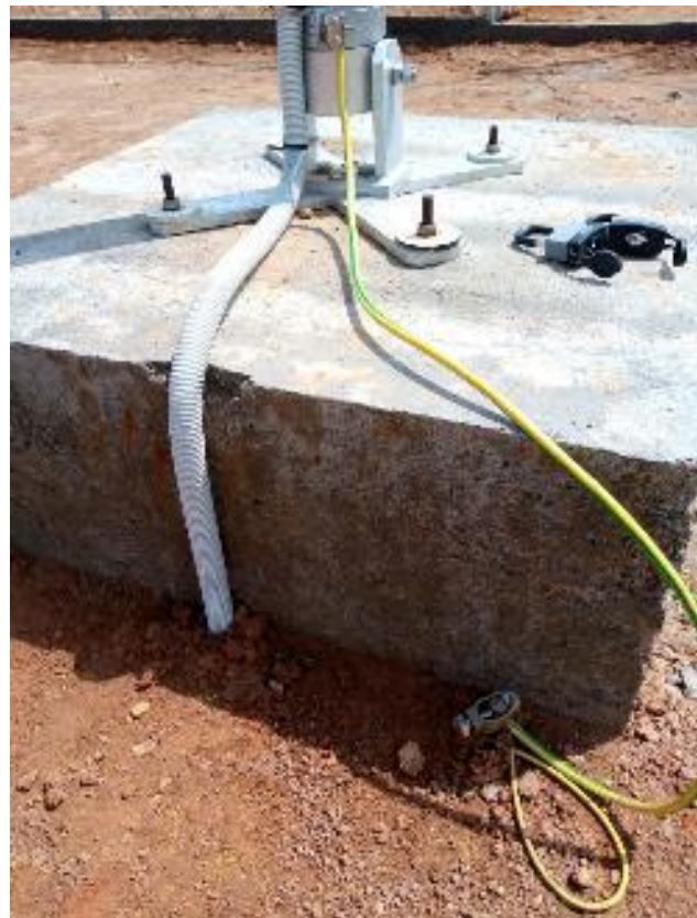
Figure 44 - Wind mast foundations, ground cable fixed to ground bolt, protective tube for wind mast cables.
