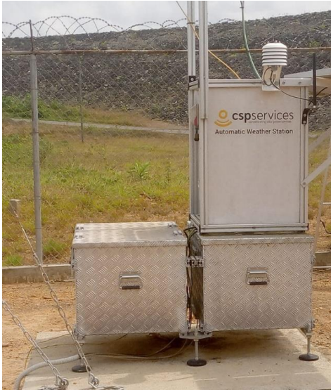
Figure 86: T/RH sensor and modem antenna on the station mounting structure
