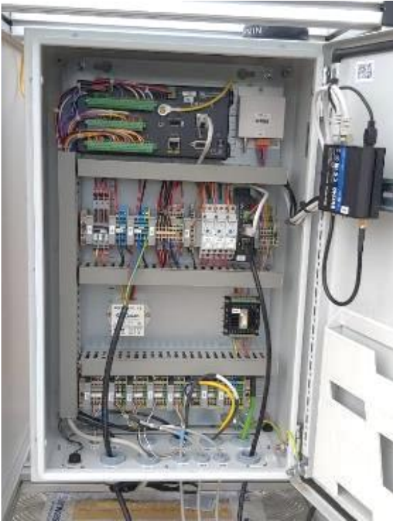
Figure 63 - Control box interior; top: datalogger; bottom: fuses and 12V circuit distribution, relays, RSI motor controller
