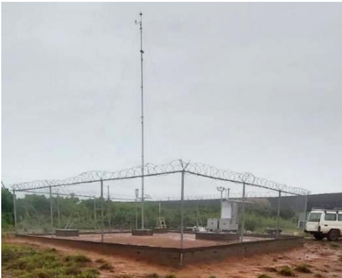
Figure 74 - Site with completed station installation as seen from south-west. Picture taken from 6.49767°N, -10.65176°E
