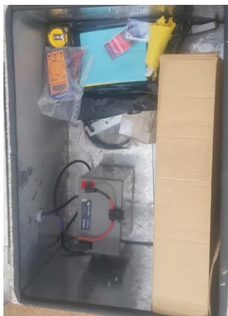
Figure 109: Battery box interior
