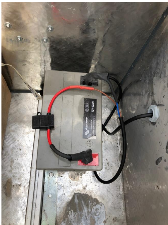
Figure 129: Battery box interior
