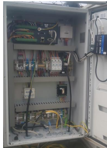
Figure 108: Control box interior; top: datalogger; bottom: fuses and 12V circuit distribution, relays, RSI motor controller and modem
