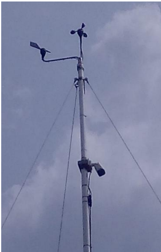
Figure 97: Wind mast top section with sensors and camera
