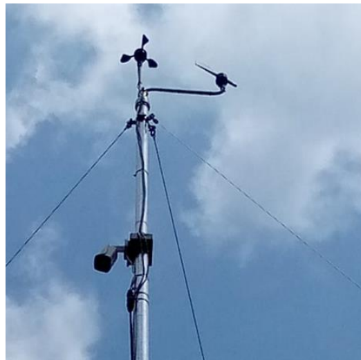
Figure 48 - Wind sensors installed on wind mast
