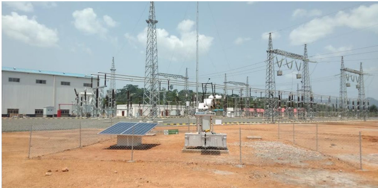
Figure 40 : Installation finale de la station vue du sud / Final station installation as seen from south.
