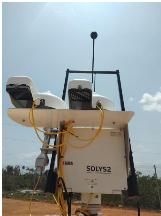
Figure 22 : Tracker installé / Installed tracker
