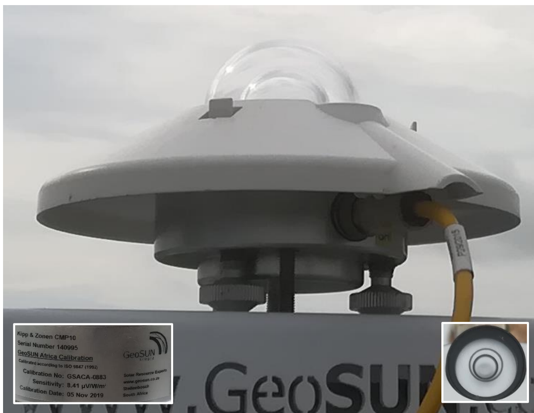
Figure 8: GHI (2) Pyranometer Installation
