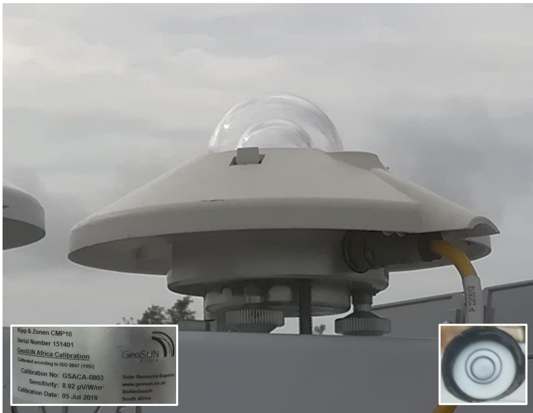
Figure 7: GHI (1) Pyranometer Installation
